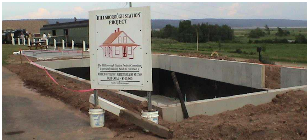
The foundation for the station, August 4. The foundation for the bathrooms is visible to the rear.
